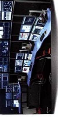
MONITORING AND CONTROL EQUIPMENT
